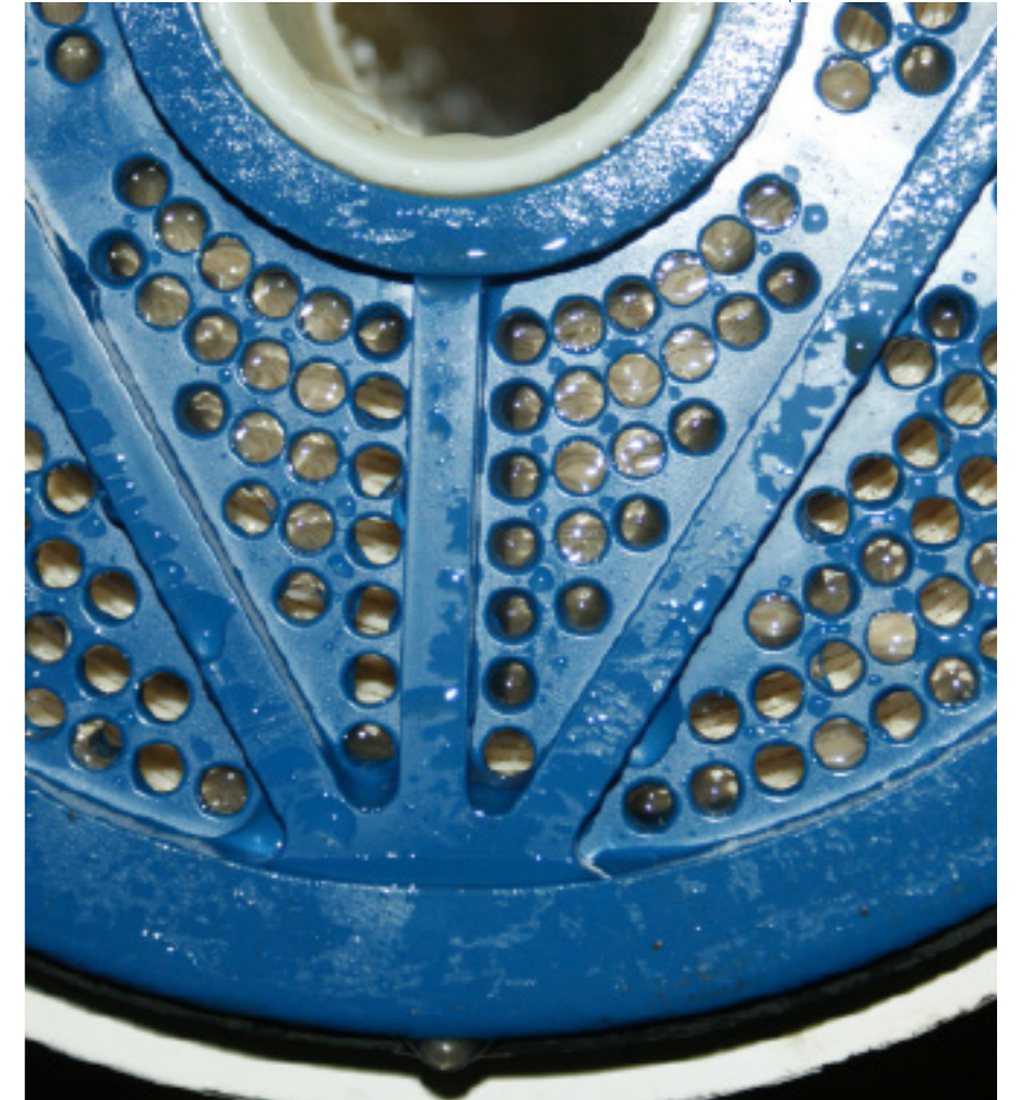
A membrane filter is used to abstract salt from the raw water
